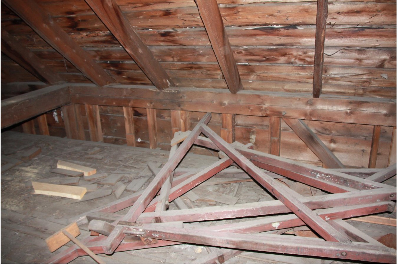
Exposed timber frame in attic and debris looking North Fishburn, S. (January 2021)
