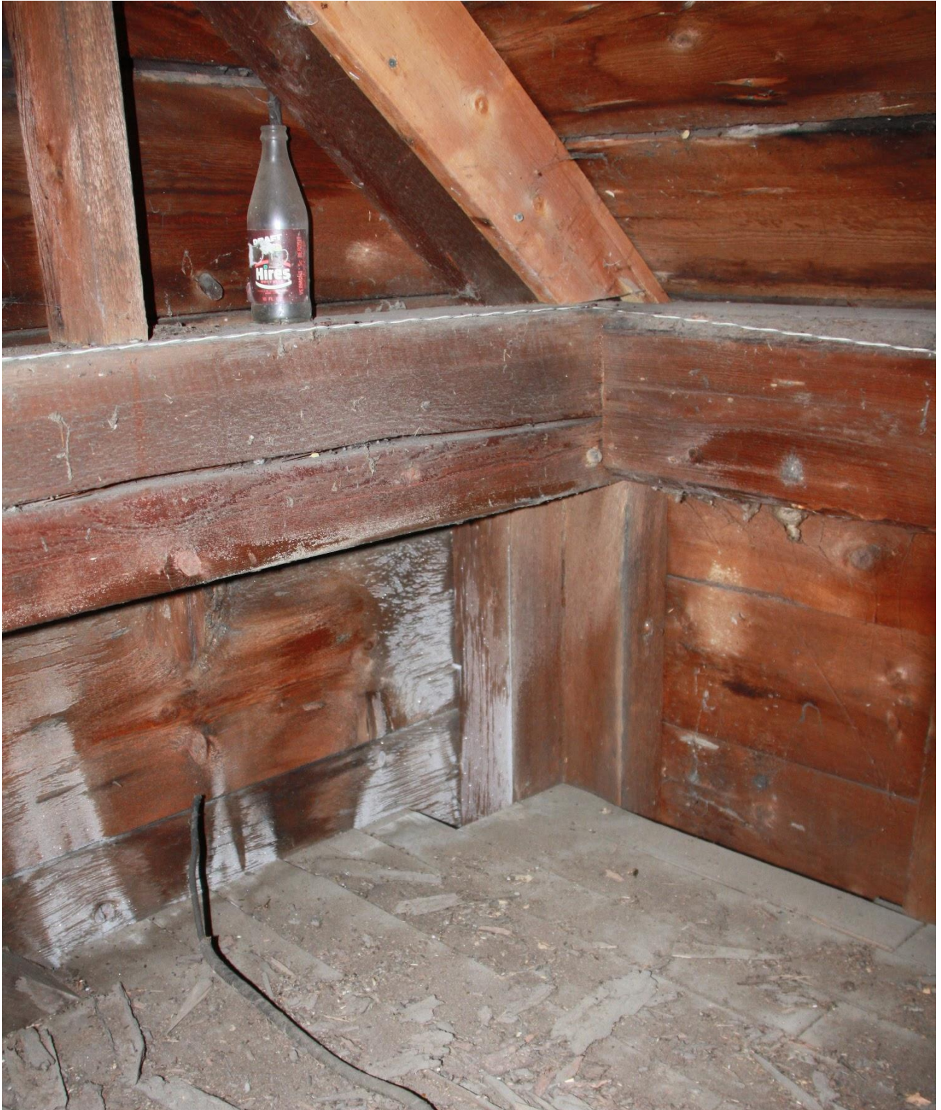
Concave column and and beam junction in attic looking northwest Fishburn, S. (January 2021)
